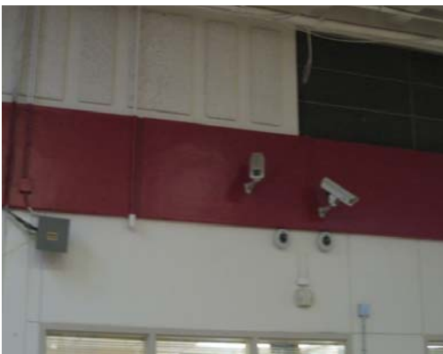
Security Cameras Installed
