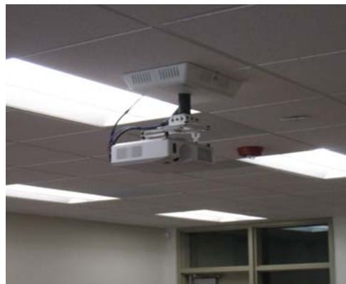
LCD Projectors Installed
